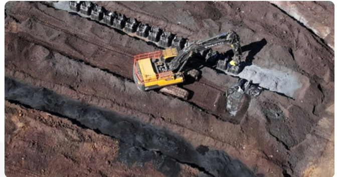
Figure 2: Aerial view of Chromium and Arsenic Contaminated Soil being Immobilised with RemBind®
